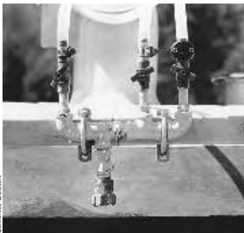
Fig. 8.25: Condenser water controls can be inexpensive needle valves. Whatever type of valve is used must allow fine control.
